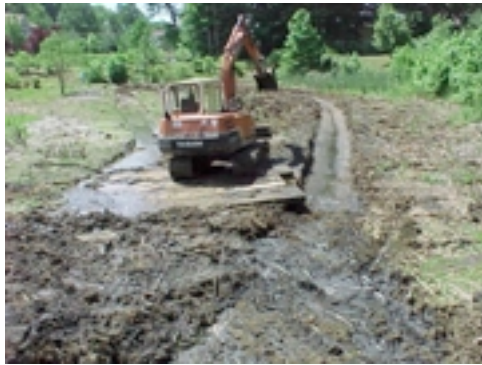
Restoring a detention basin after years of neglect requires heavy equipment and is expensive. The above basin was full of water and more than two feet of mud buried the low flow channel.
